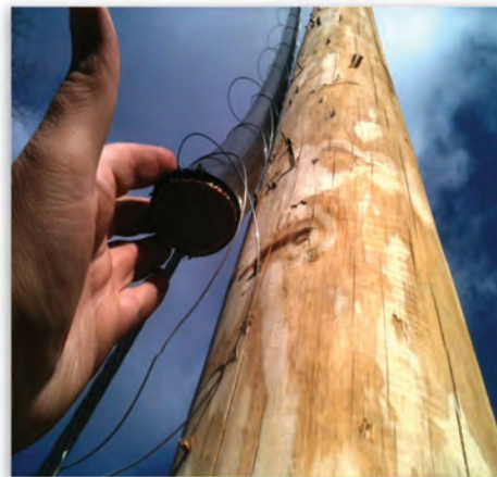
A Frontier Communications’ employee surveys the damage left behind by copper thieves in West Virginia. The company has replaced 38,000 feet of stolen cable since August 2011.
