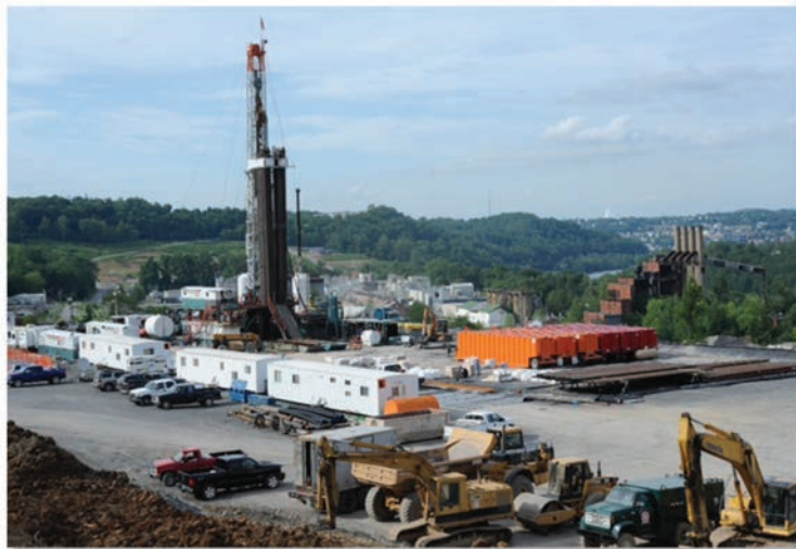
Northeast Natural Energy’s shale gas drilling operation is located in the Morgantown Industrial Park in Monongalia County, W.Va.
